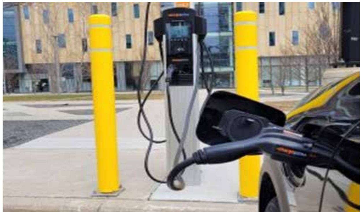
EV charging stations at Sheridan College – Hazel McCallion Campus
