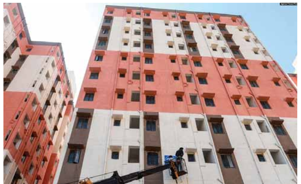
A construction worker fixes a window in a housing complex for people under the economic category of Below Poverty Line in Kolluru, on the outskirts of Hyderabad Feb. 1, 2022.
