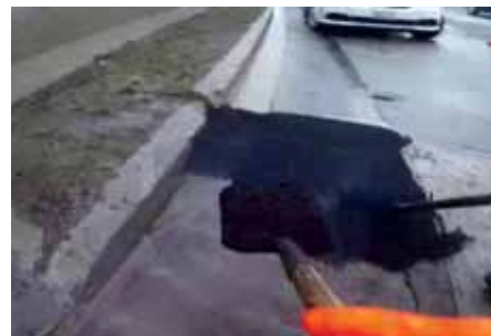
City crews fill potholes with cold-mix concrete in the winter, then apply hot-mix concrete in the summer to provide a more permanent fix. (Paul Borkwood/CBC)
